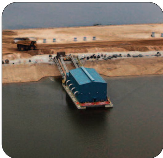
Water reclaim barge pump house in operation
